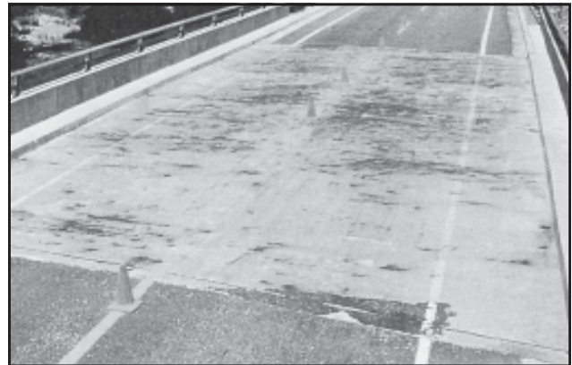
Steel corrosion on a bridge deck
